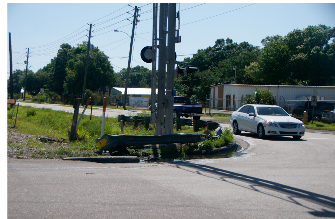
Damaged guardrail caused by turning trucks at the intersection of Wabash Avenue and Olive Street in Lakeland
